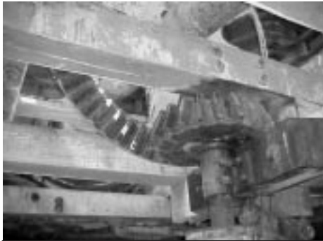
Rusted mechanical system of the South Windmill will undergo restoration.
